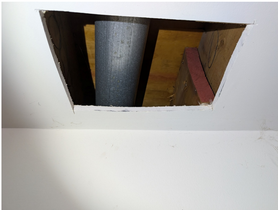
Joists Bearing on Top of Wall
